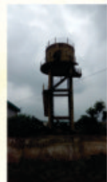
OVERHEAD WATER TANK Capacity 50000 L
