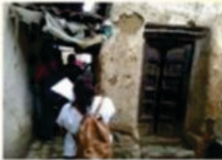
BAD WALL CONDITION
